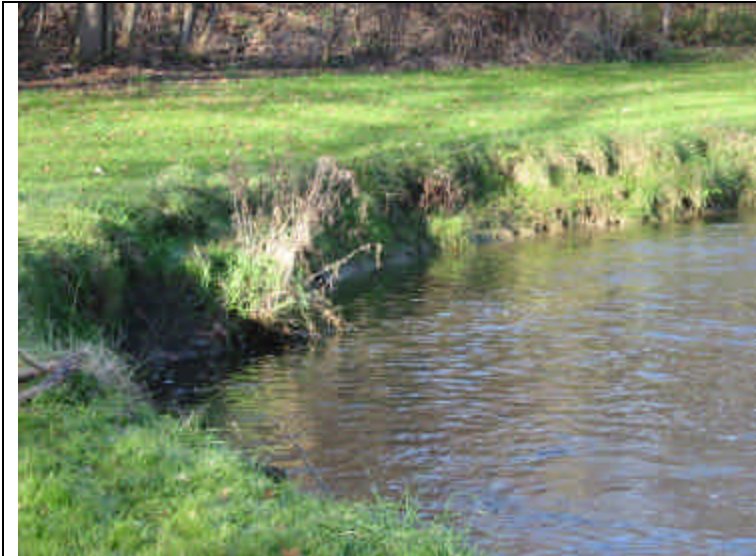
Erosion on south bank of Oatka Creek at 1198 Quaker Road. Note slumping from undercutting of clay bank.
