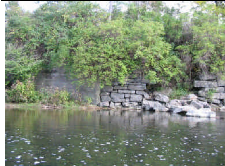
Failing retaining wall at southwest quadrant of Rochester & Southern Railroad bridge over Oatka Creek
