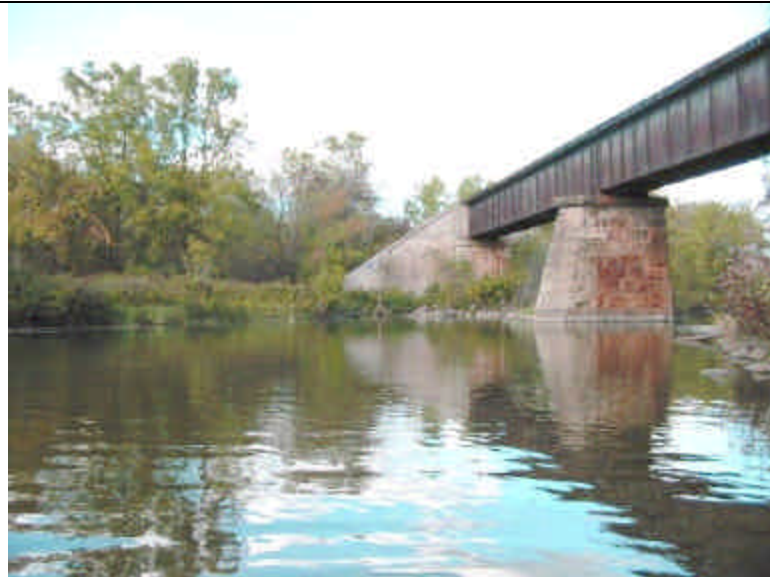
View of northwest quadrant of bridge. Current hits abutment at near right angle, creating scour hole at northwest quadrant.
