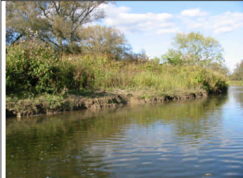
West/north bank of Oatka Creek near railroad bridge (typical). Note exposed soil in scour areas.
