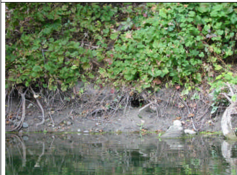
Photo 3. Bank conditions typical of north bank approximately 1500 feet east of Munson Street bridge. Note muskrat hole in bank just above water level.
