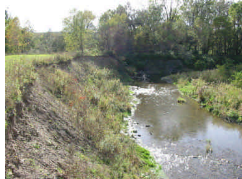
View of Oatka Creek exposed soil bank near Station A0+600, looking northwest along channel.
