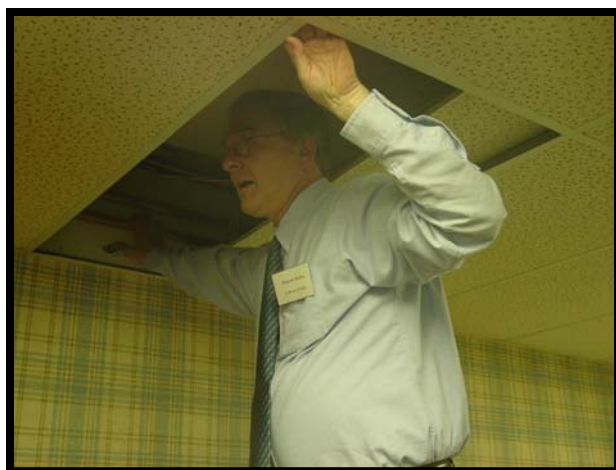
Wayne Balas, CJ Brown Energy, inspects the ceiling of Victor Village Hall for insulation
